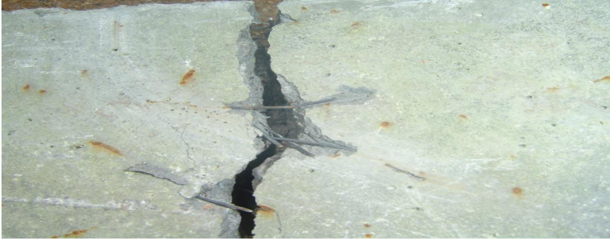
Fig 21: Failure pattern in concrete beams after undergoing flexure test
