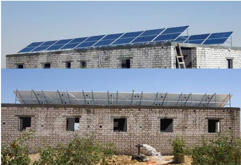
Fig. 4: general site of PV pumping system.
